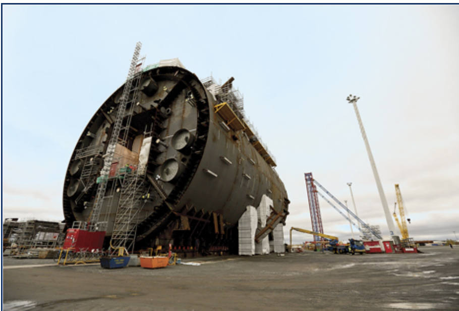
Fig. 1. The truss spar for Anadarko's Lucius project in the Gulf of Mexico is under construction at Technip's Pori, Finland shipyard. Photo courtesy of Technip.
